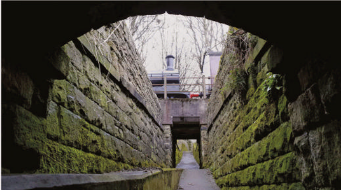
A stone-lined, sunken path might add a bit of interest and save the space needed for slope-sided cuttings. This is Keighley, West Yorkshire, where a stream has been culverted and turned into a path (with quite low head-height under the old bridges).
