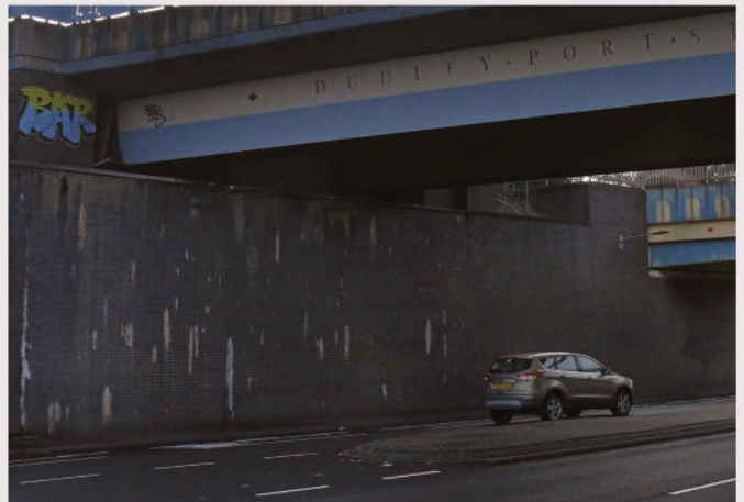
Something a bit gritty and urban; Dudley Port, West Midlands, and a huge, heavy-duty brick-faced wall carrying the main line and a canal over the road. Of particular interest are the limescale deposits and water staining, and the graffiti, which must have been a hell of a job for a precariously-dangling artist.
