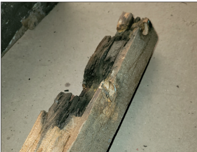
Extensive brown rot, initiating from the upper plank edge, can be seen in this inner surface of courbaril planking.
