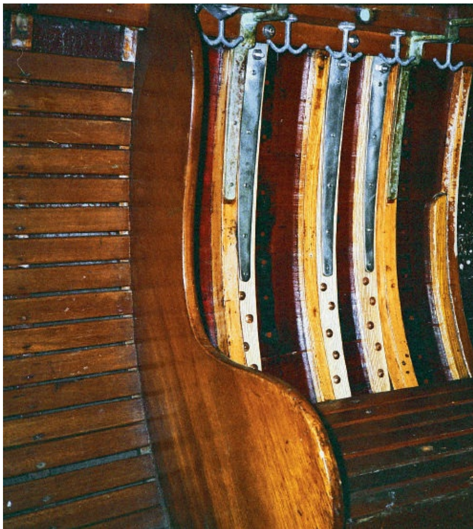
FIGURE 192 } Chain plate mounted on wooden plates. To the right are wood frames that have been sistered.
