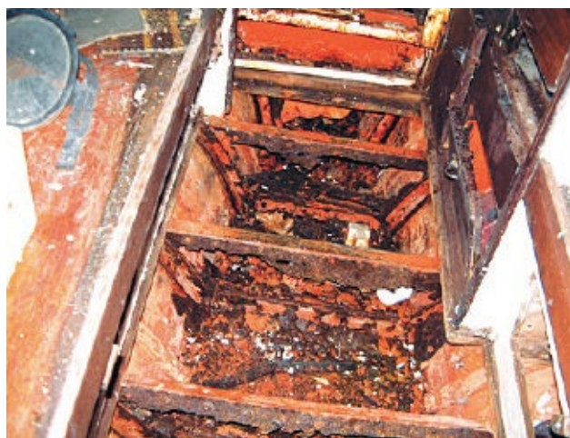
FIGURE 114 } Rusty floors. This renovation has to begin with a broom and a shovel.
