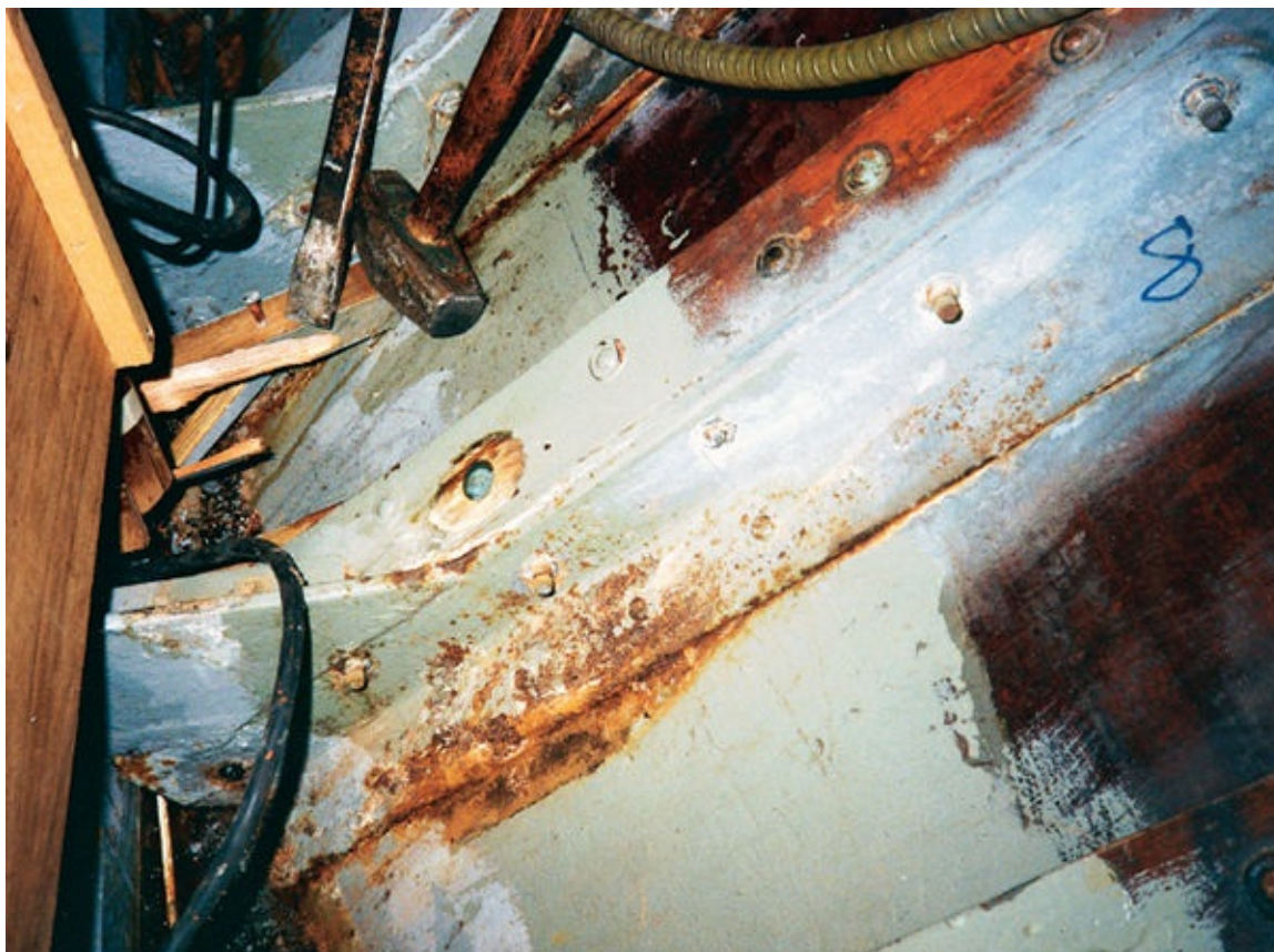
FIGURE 38 } Nail sickness in wood from a copper nail in contact with a galvanized bolt in the rib.
