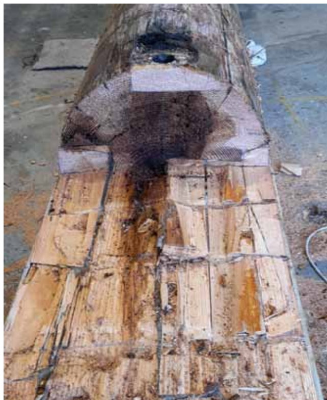
FIGURE 2 – Extent of degradation of timber at deadeye.
