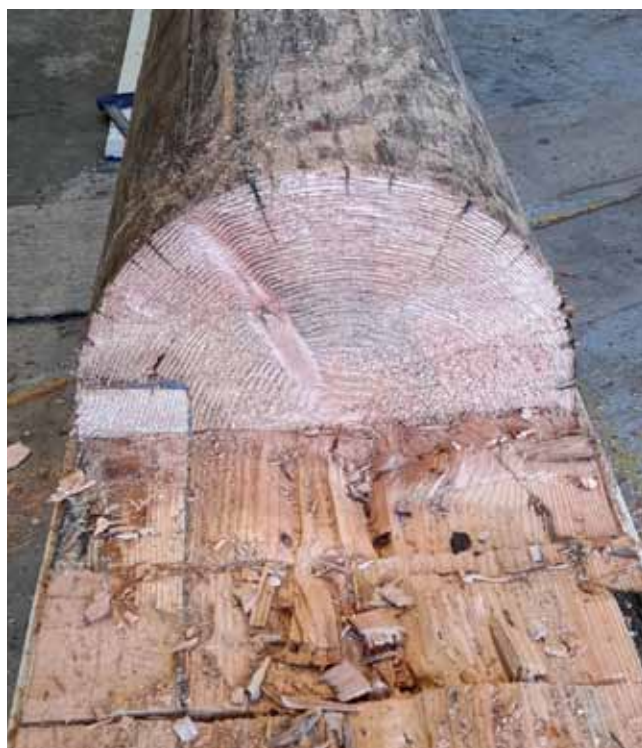
FIGURE 4 – Stable Oregon demonstrating extent of cracking.
