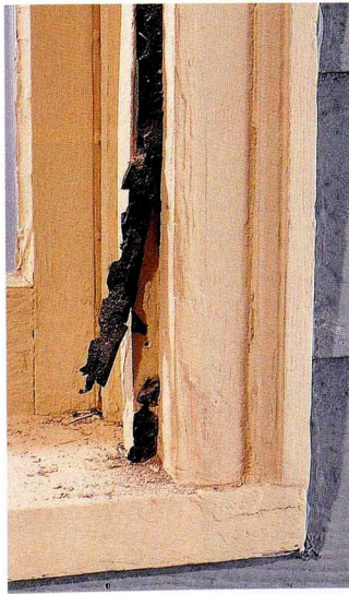
Weatherstripping and insulation may begin to deteriorate. Telltale signs include crumbling foam or rubber.
