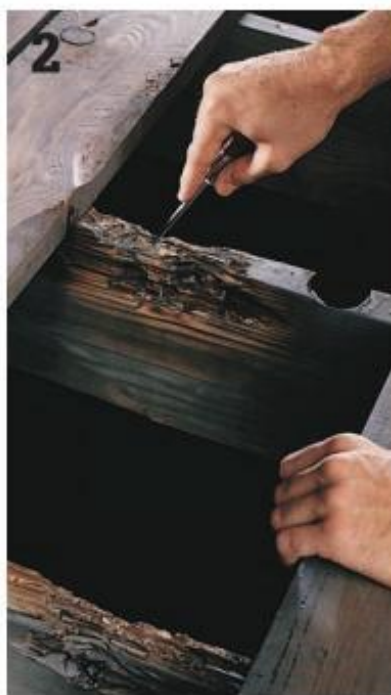
2 Inspect the underlying joists for signs of rotted wood. Joists with discolored, soft areas should be repaired and reinforced.
