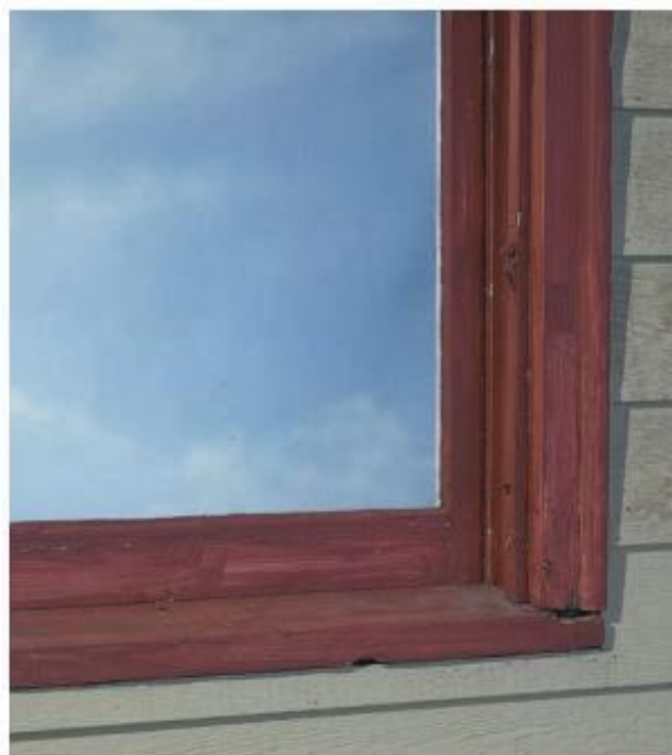
Check window and door trim for rot , especially on horizontal surfaces and at joints. Try to make repairs without removing the trim.
