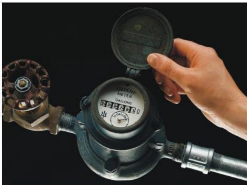
Water meter and main shutoff valves are located where the main water supply pipe enters the house. The water meter is the property of your local municipal water company. If the water meter leaks, or if you suspect it is not functioning properly, call your water company for repairs.
