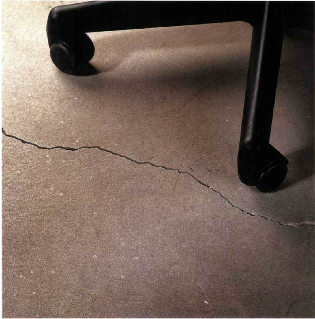
Although concrete is very durable , it can still be chipped by heavy objects or cracked due to abrupt changes in temperature or house shifting.
