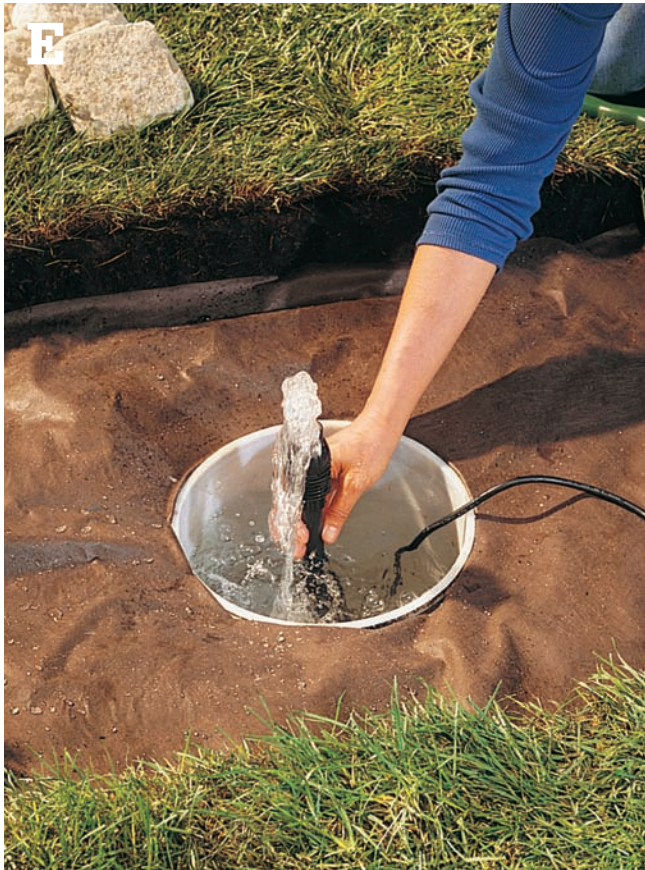
E Fill the basin with water and adjust the flow valve on the pump to create a pleasing effect.
